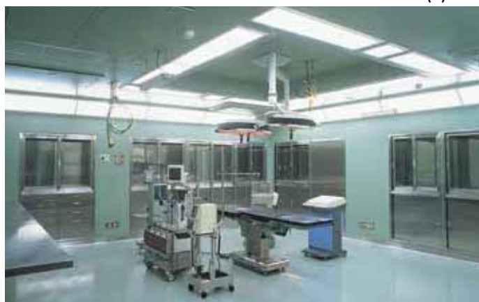
Installation example (in a medical facility)
